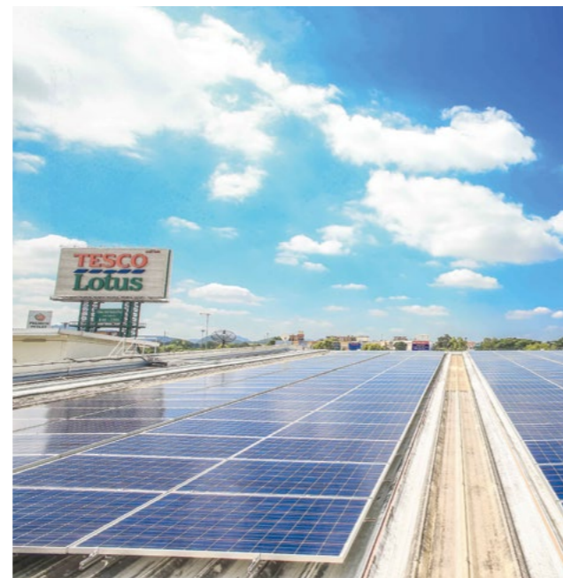
In Thailand we have fitted 36 sites with solar panels as we look to source 100% of our Group electricity from renewable sources by 2030.
